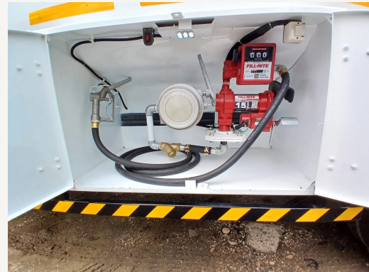
Components fitted to a tank unit
